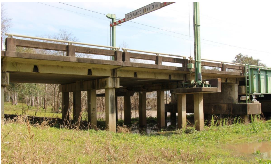
Historic Fabric Photo 2: Concrete substructure and concrete approach spans with concrete and metal tube railing northeast of the main swing span; also showing the traffic barrier gate and towers.
