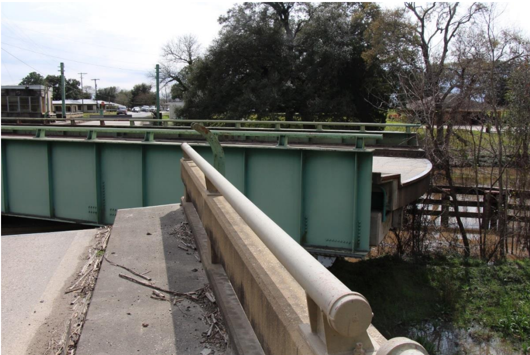
Condition Photo 18: Steel plate girder swing span hitting vegetation located west of the bridge. Also note the debris along the approach span shoulder and the sidewalk and the paint system failure.
