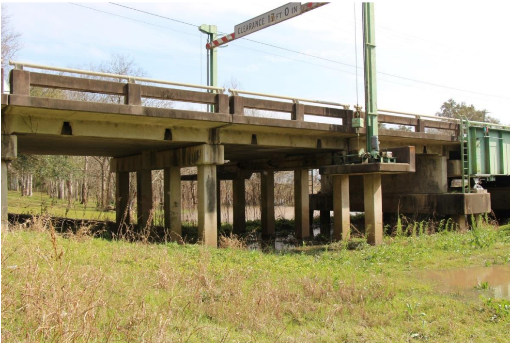
Condition Photo 14: Water staining on concrete slab and bents on the approach spans, typical condition.
