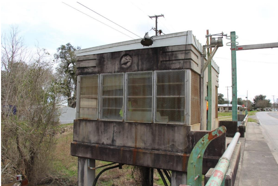
Condition Photo 20: Operator's house, north walls, windows, and metal protective screening over windows, looking south.
