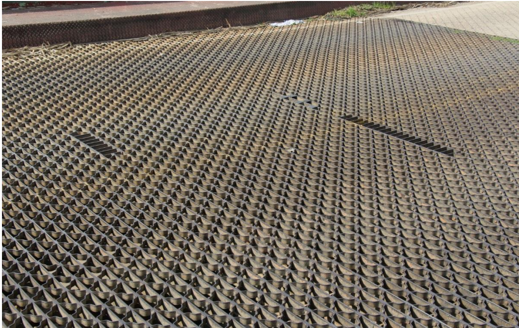
Condition Photo 5: Open metal grid deck condition showing repairs on swing span.
