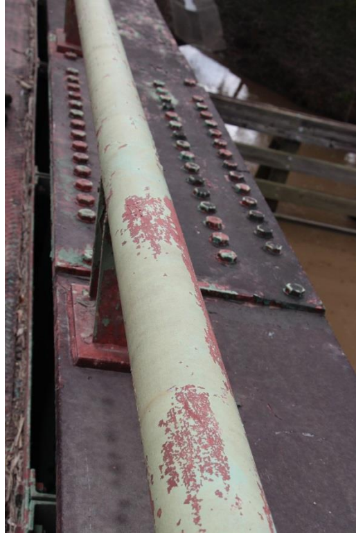
Condition Photo 15: Main span longitudinal steel girder and steel railing paint failure.
