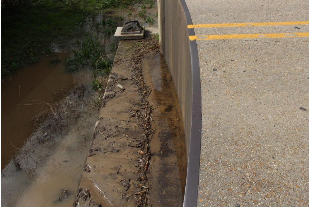
Condition Photo 19: Drift, water, and debris build-up at pier 3 for the swing span bearing seat.
