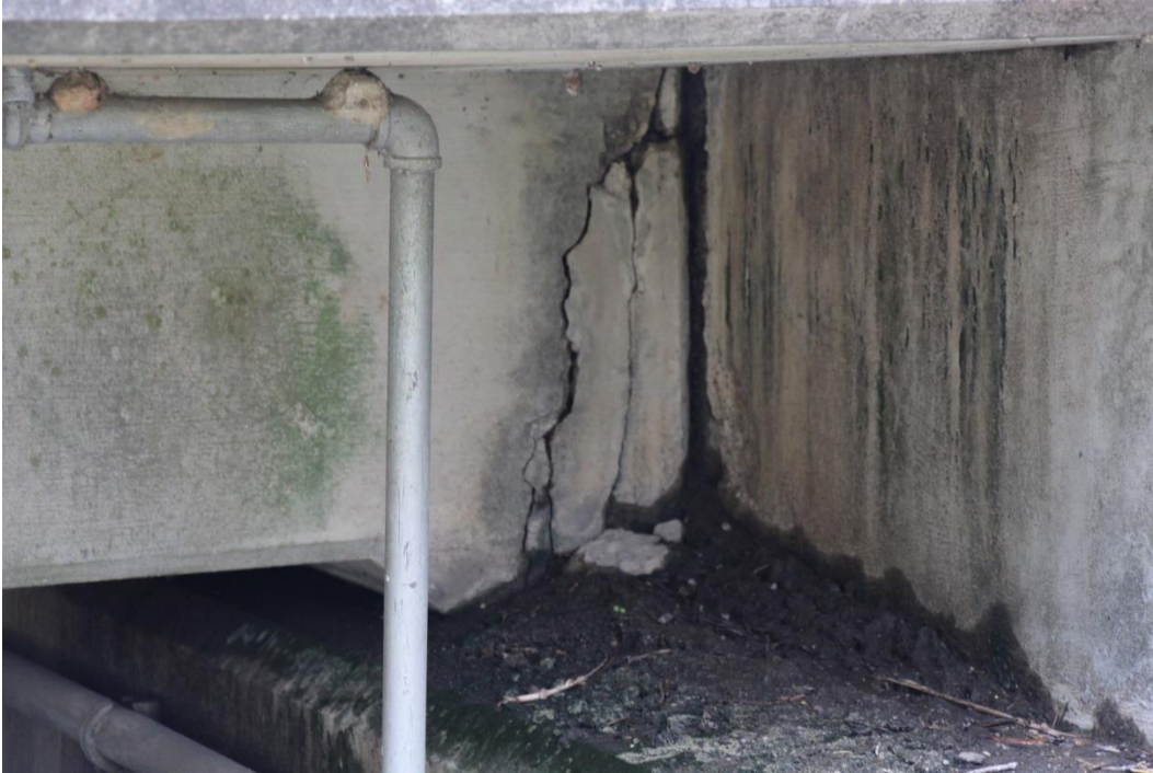
Condition Photo 9: Crack in haunch of concrete deck slab at the end bent 1.
