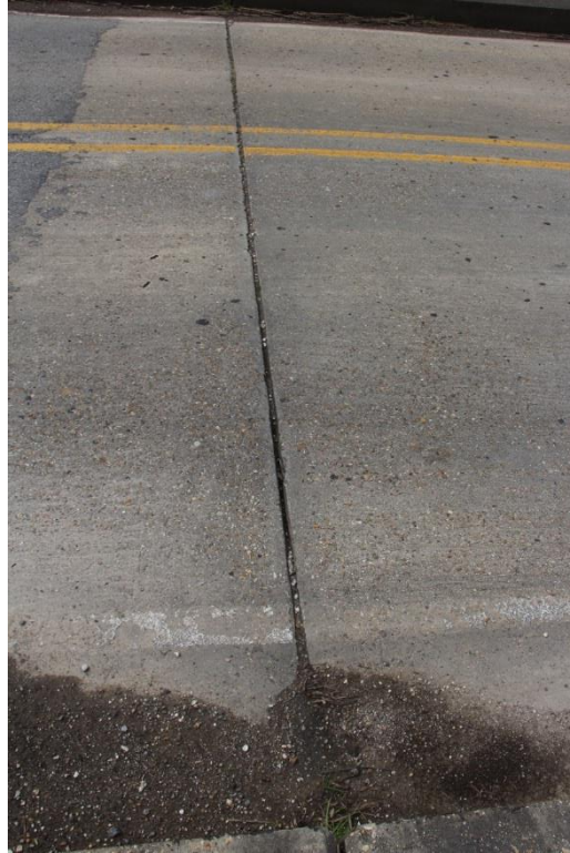
Condition Photo 7: Deck expansion joint and shoulder full of debris, typical for approach spans.
