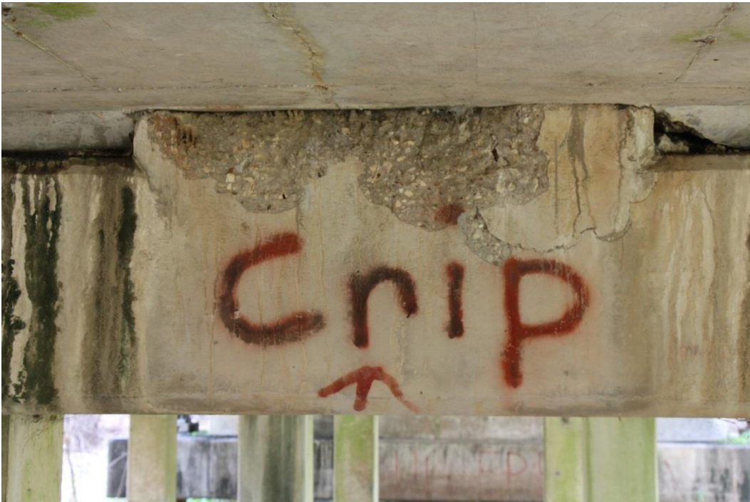
Condition Photo 12: Bent 10, spalled concrete bent cap where the deck and haunch meet at the bent cap; also note graffiti on bent cap.
