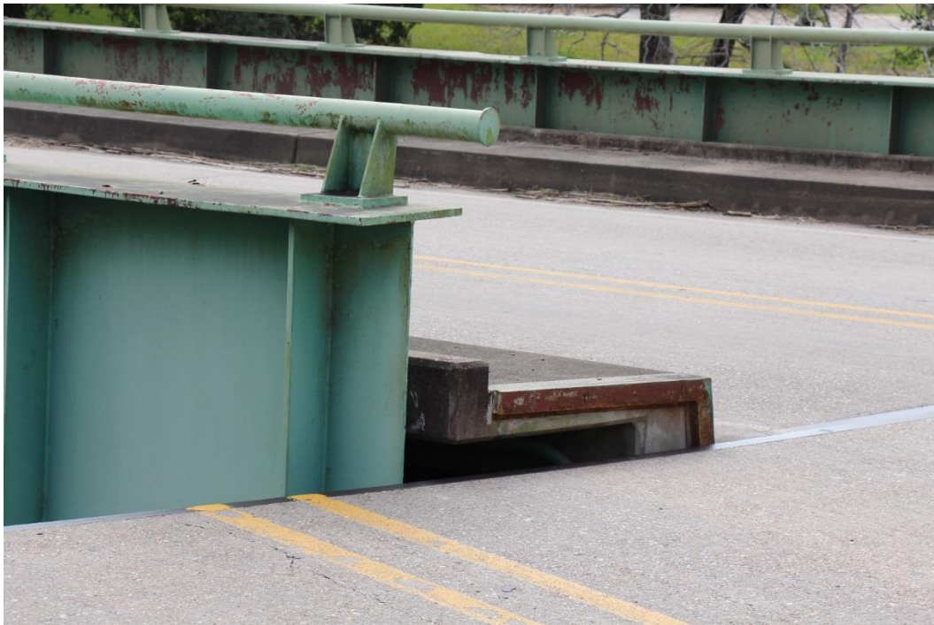
Condition Photo 16: Paint failure on the girders, railings, and sidewalks of the swing span.
