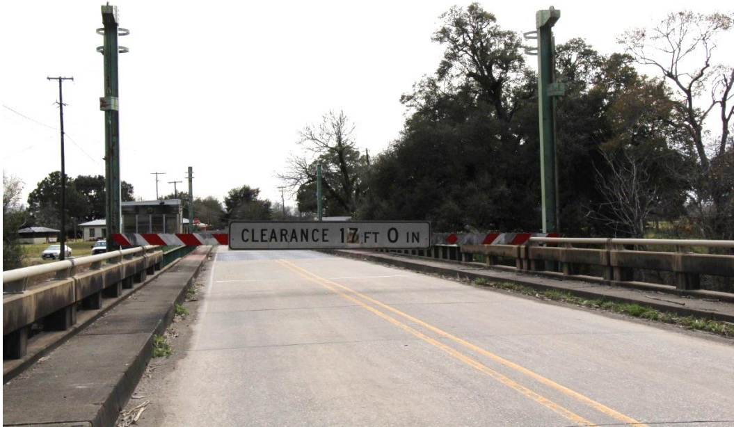
Condition Photo 3: North traffic barrier gate with towers and vertical clearance sign, looking south.
