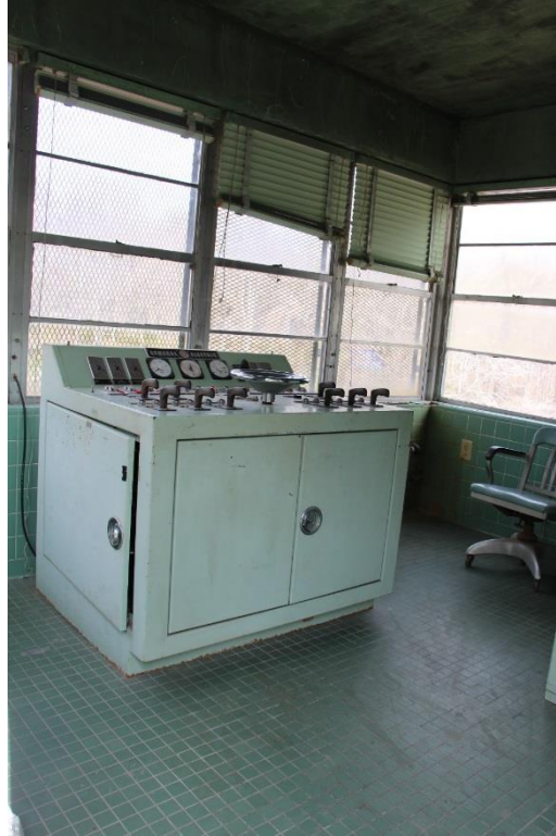
Condition Photo 21: Control console and tile floor in the operator's house.
