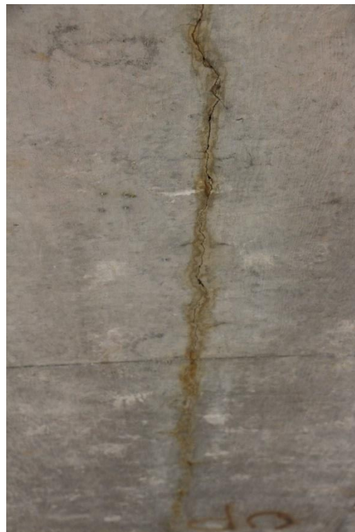
Condition Photo 6: Typical concrete slab approach span cracking and efflorescence on the underside of the slab.
