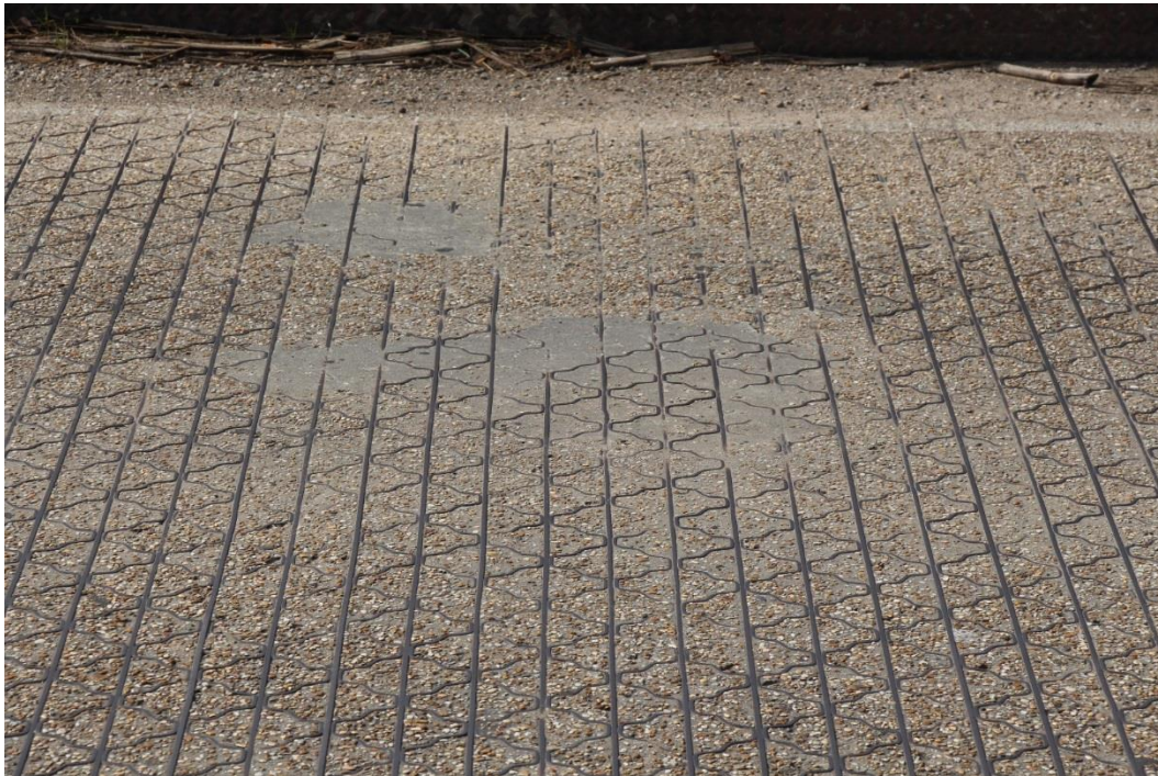
Condition Photo 4: Concrete-filled metal grid deck wear and patched areas on swing span.
