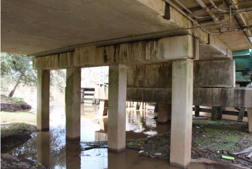
Condition Photo 13: Concrete bent cap and columns exhibiting water staining, typical condition.
