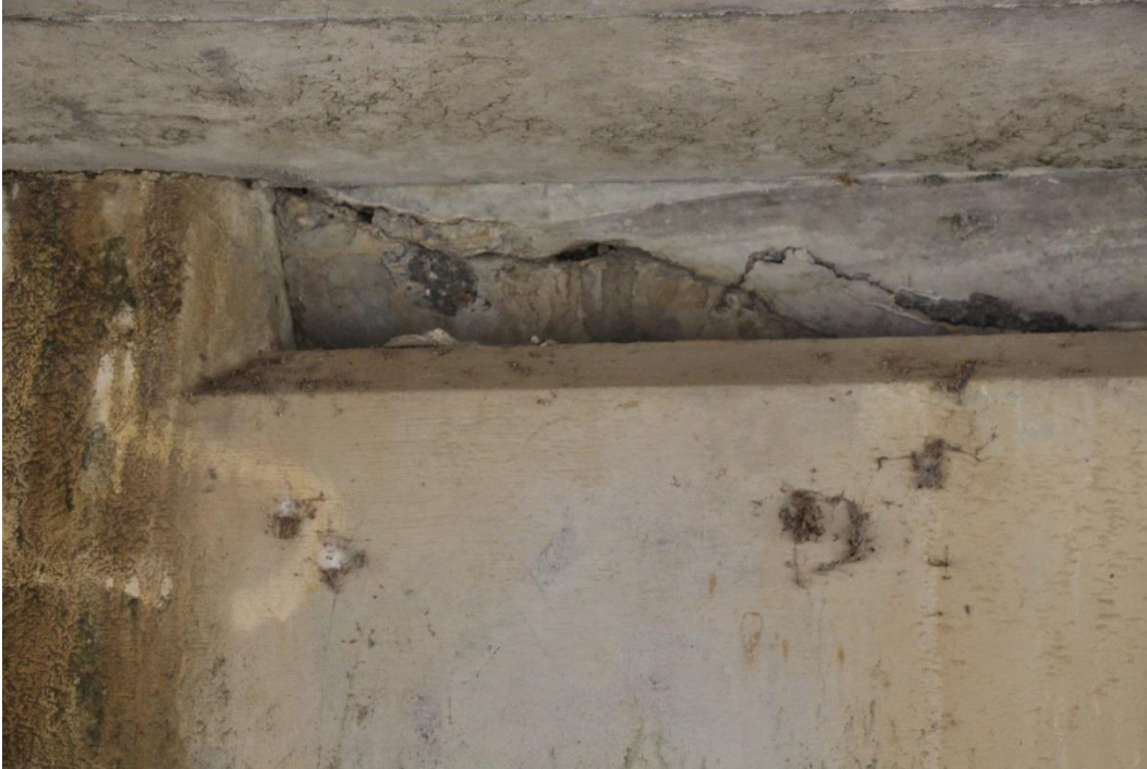
Condition Photo 11: Spall at the concrete deck slab where the deck and haunch meet at bent 4.
