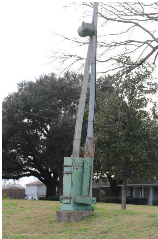
Condition Photo 22: Traffic gate exhibiting minor paint failure.
