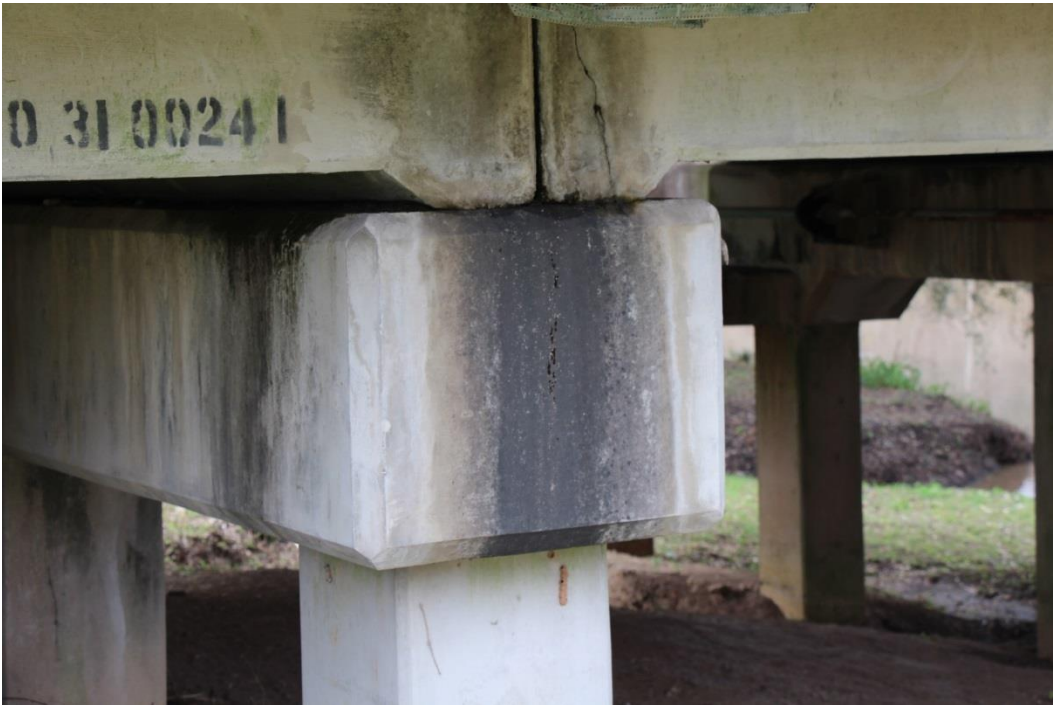
Condition Photo 10: End of concrete bent cap water staining and crack in concrete deck slab haunch.
