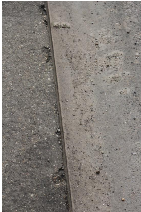
Condition Photo 8: Spalling of the concrete joint in approach span concrete deck at concrete approach slab at end of bridge.
