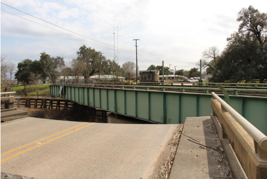
Condition Photo 17: The opening of the steel plate girder swing span. Also note the debris along the approach span shoulder and the sidewalk and the paint system failure.
