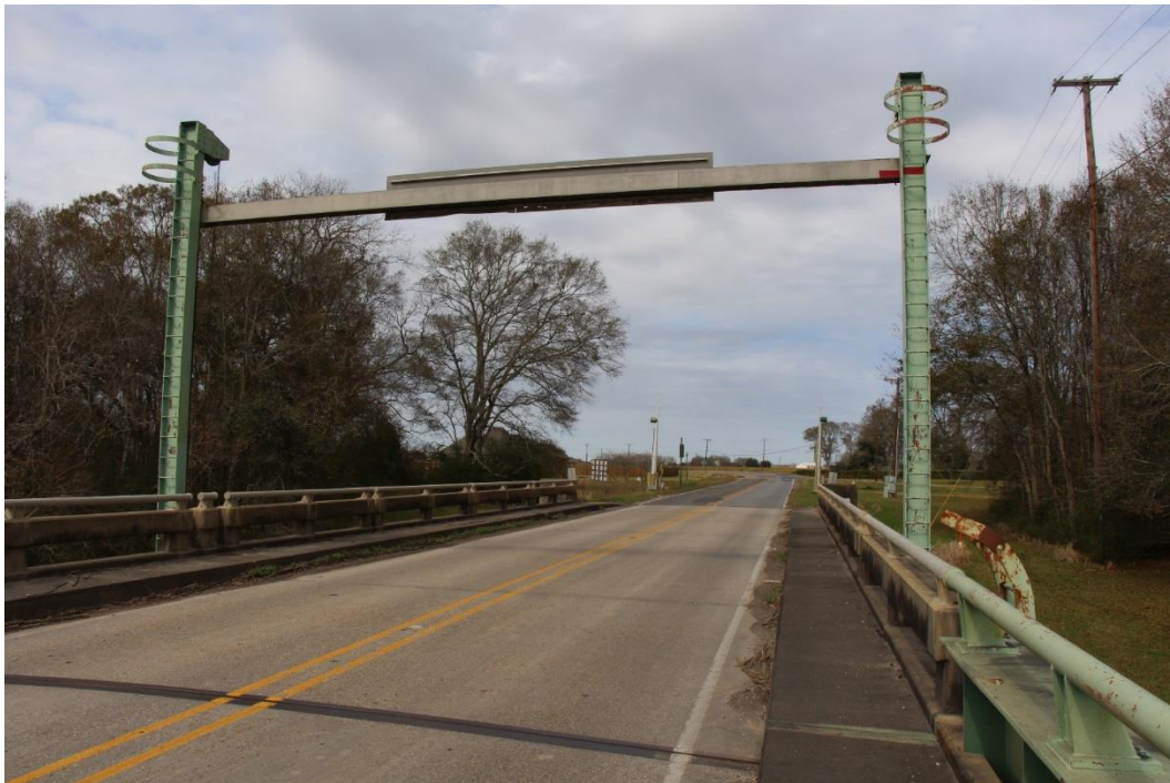
Condition Photo 2: Northerly concrete approach spans and traffic barrier gate, looking north toward north end of bridge.
