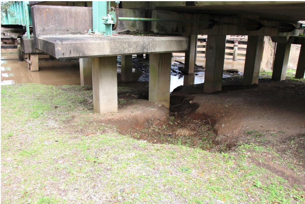
Condition Photo 24: Bent columns exhibiting scour at the columns of bent 3.
