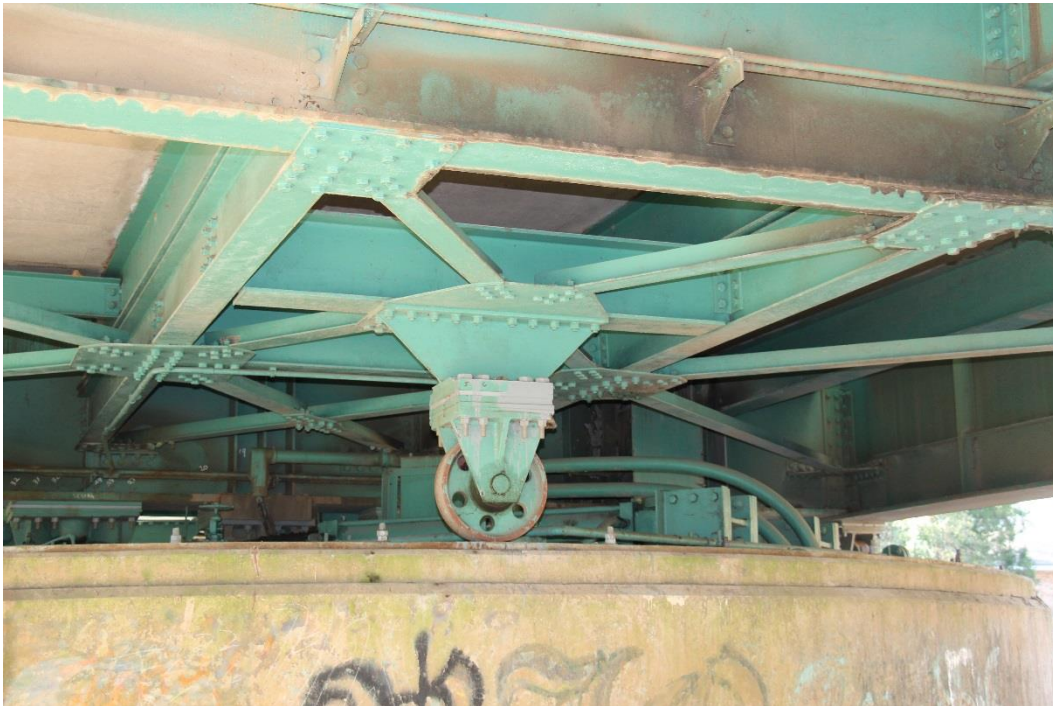
Character-defining Feature Photo 3: Design and construction of the center-bearing turning mechanism. This roller-and-track system guides the motion of the bridge when it opens and closes.
